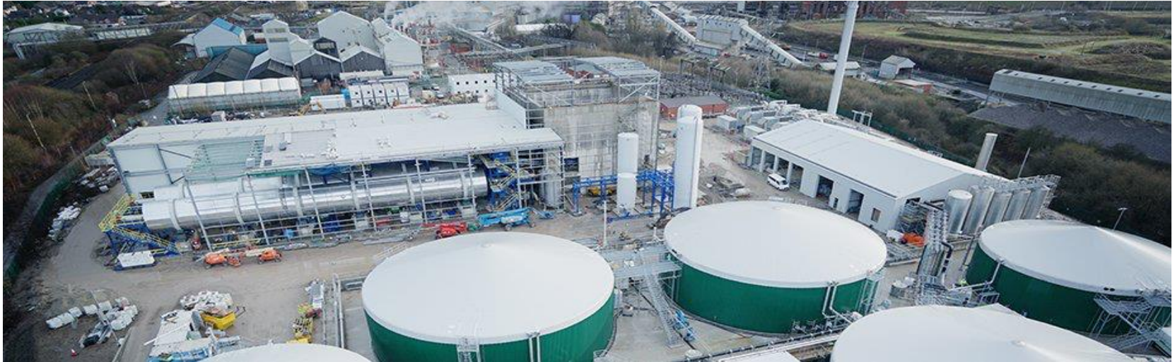
Renescience waste conversion plant Northwich, England
