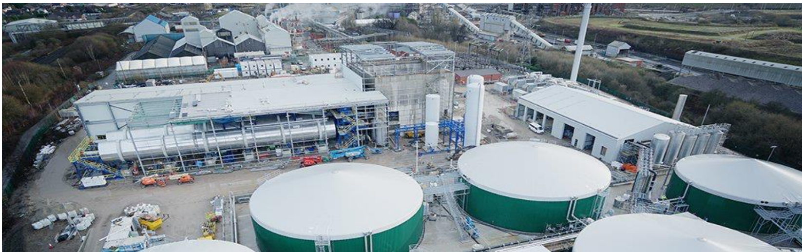
Renescience waste conversion plant Northwich, England
