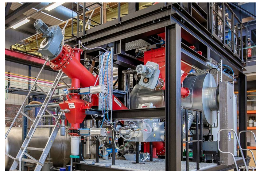
1 MWth demo two-stage gasification installation at DNV in Groningen
